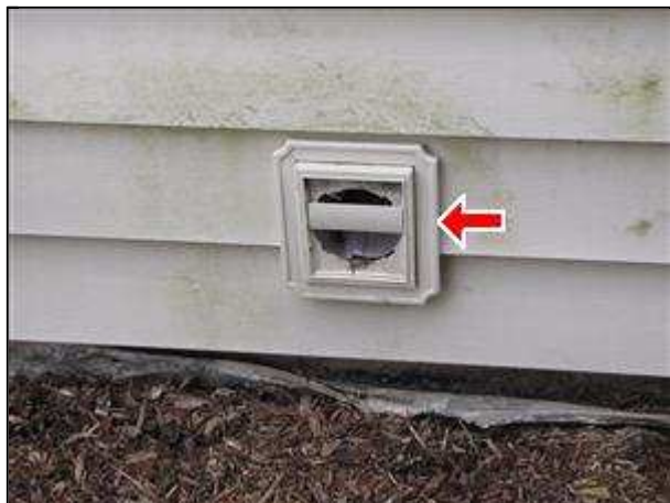
9.3 Item 1(Picture) Replace dryer vent damper to prevent entry of mice.
