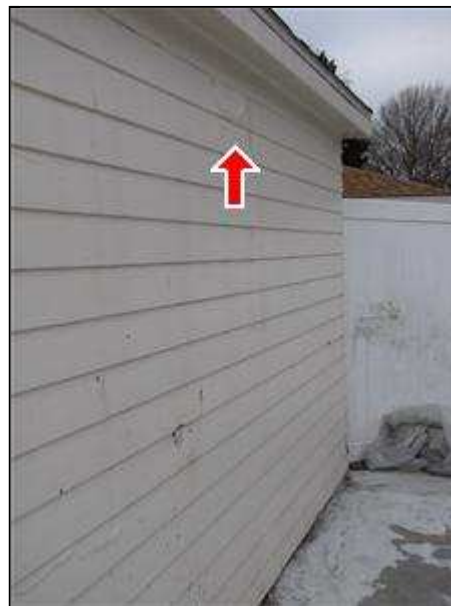
3.1 Item 2(Picture) Paint on garage has large bubbles.
