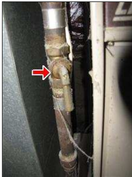
8.0 Item 2 (Picture) Gas valve for furnace.
