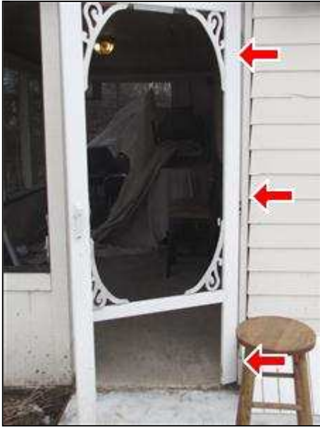
3.3 Item 1(Picture) Screen door to garage screen room needs replacement.
