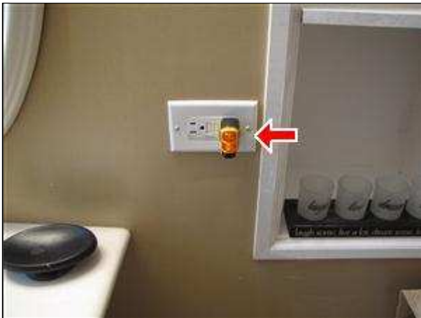
7.5 Item 3(Picture) Gfci receptacle in lower level washroom failed testing.
