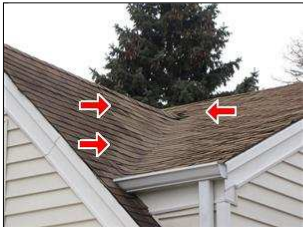
1.0 Item 1(Picture) Shingles are beginning to lift at peak of roof.
