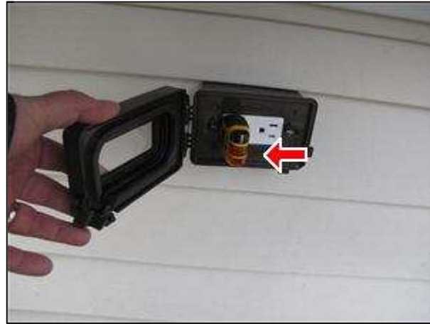
7.3 Item 2(Picture) Exterior receptacle on East elevation not working and must be replace with a gfci type.
