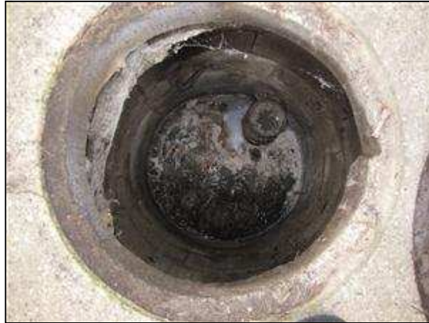
6.0 Item 2(Picture) Inspector recommends cleaning of catch basin in rear yard.
