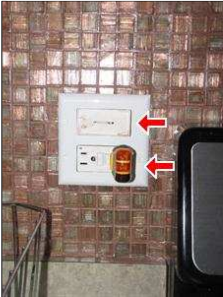
7.5 Item 1(Picture) Gfci receptacle near kitchen sink not working. Dimmer switch for can light not working.
