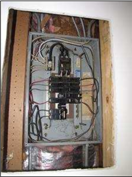
7.6 Item 1(Picture) Electrical panel west wall of laundry room.
