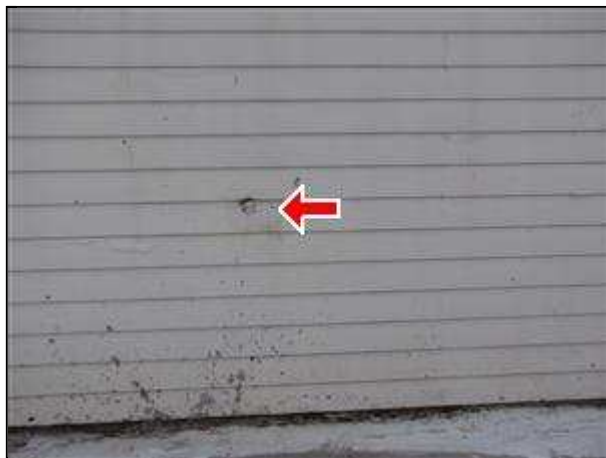
3.1 Item 1(Picture) Hole in siding on north elevation
