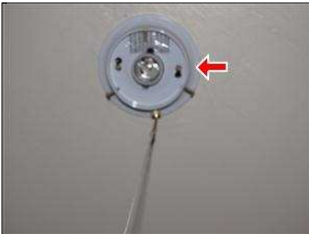
7.3 Item 3(Picture) Closet light is missing a globe.
