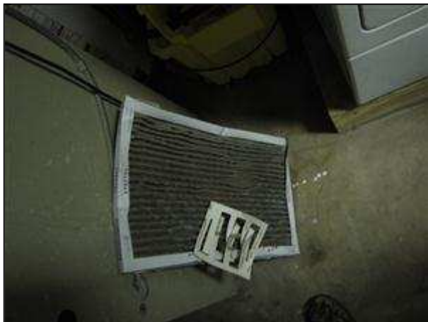
8.0 Item 1 (Picture) Furnace filter is clogged and sucked into fan. Filter that was installed is of the wrong size. the correct size is 16X25X4
