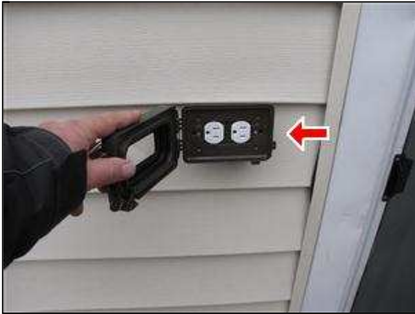
7.3 Item 1(Picture) Exterior receptacle on west elevation must be replaced with a gfci type.
