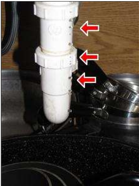
6.0 Item 3(Picture) Kitchen sink drain is leaking.
