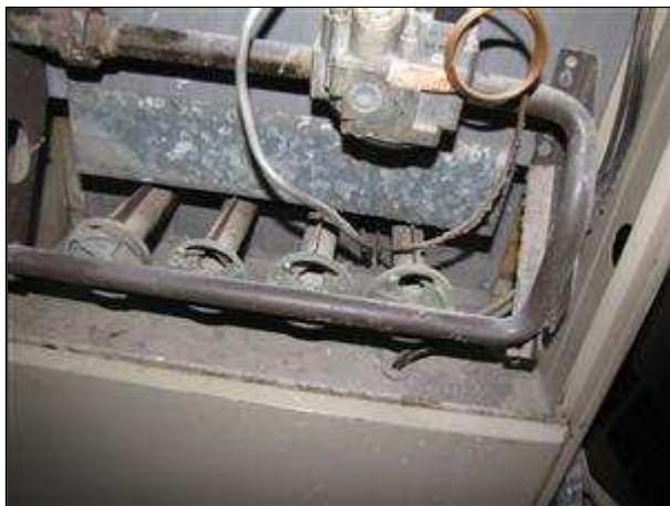
8.0 Item 3 (Picture) Inspector recommends cleaning and maintenance of furnace by qualified hvac contactor.
