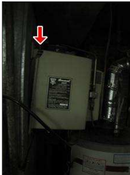
8.1 Item 2(Picture) Humidifier mounted to furnace plenum has been broken at its mounting.
