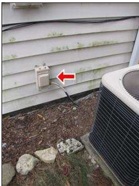
8.6 Item 1(Picture) Electrical service disconnect. Lift cover and pull out switch.Never lock this.
