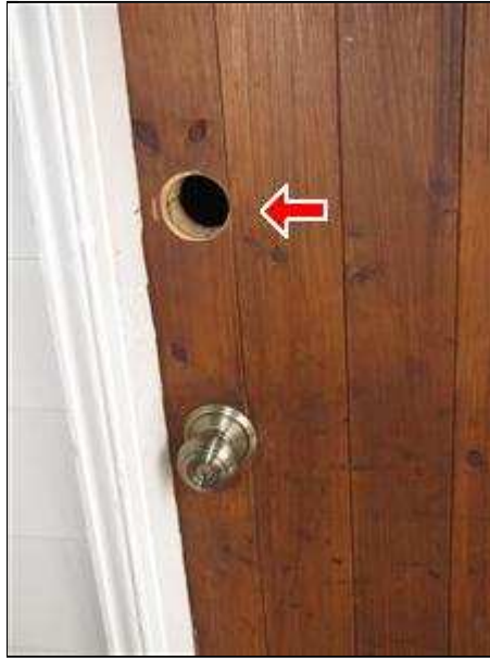
3.3 Item 2(Picture) Garage entry door missing dead bolt lock
